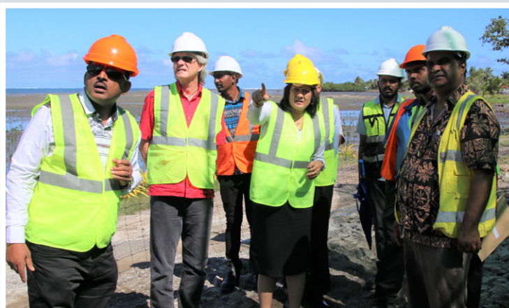
Education Minister Rosy Akbar visits FNU capital project sites with FNU Chancellor and Chair of Council Dr Rajesh Chandra and VC Professor Nigel Healey and receives construction updates from contractors.
