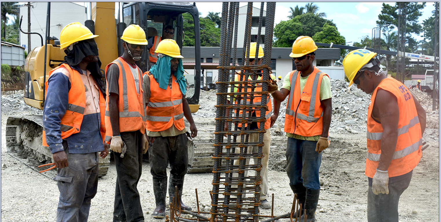
Construction work on the four-storey CBHTS building underway at FNU Nasinu Campus
